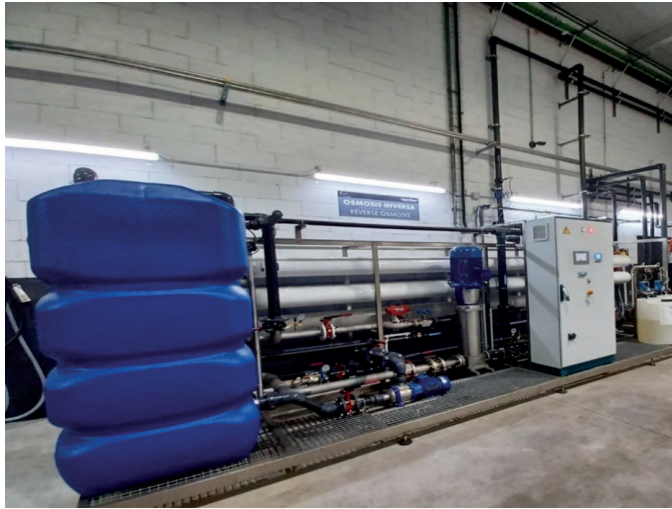
IMAGE 1: Nalco Water membrane system treating effluent water.
